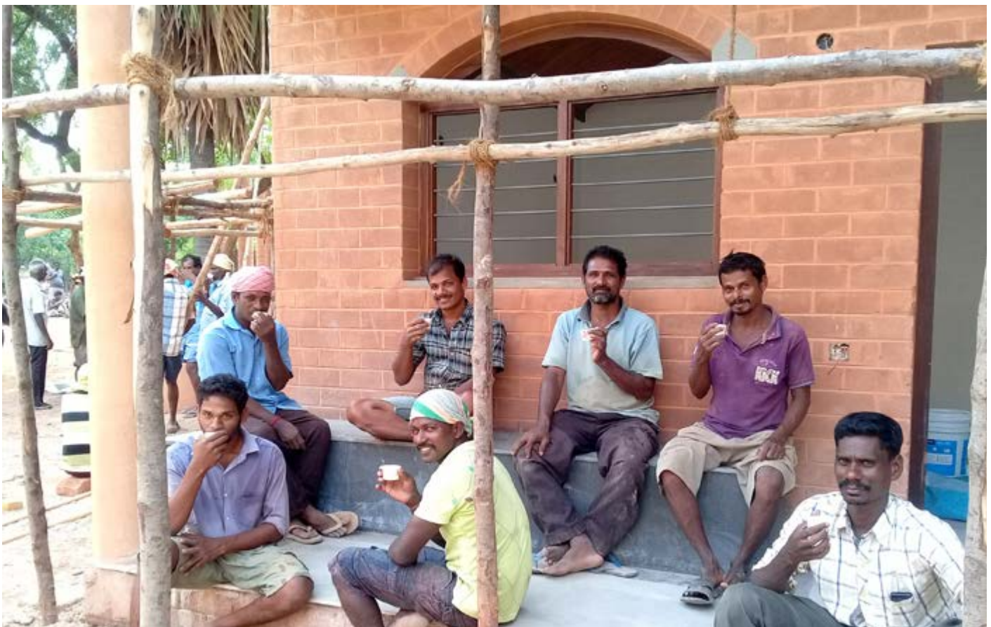
A warm thanks and congratulations to the crew of Sharanam who have been working with dedication and skill to complete the double-story units, the PEC road, and the conference hall. Thank you!
