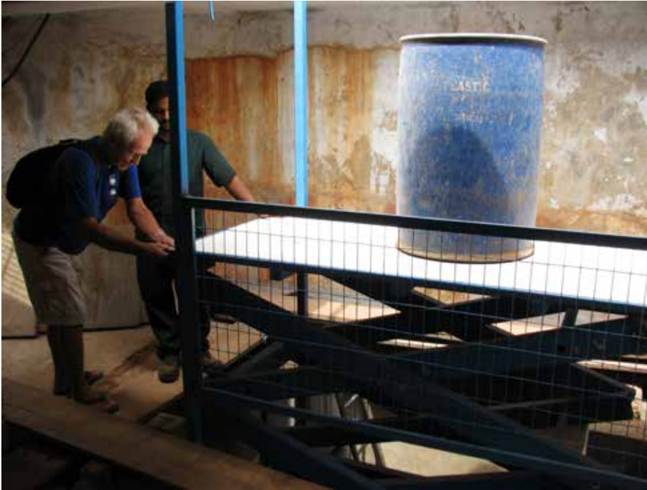
The hydraulic lift for garden equipment being installed in the underground Tools Center
