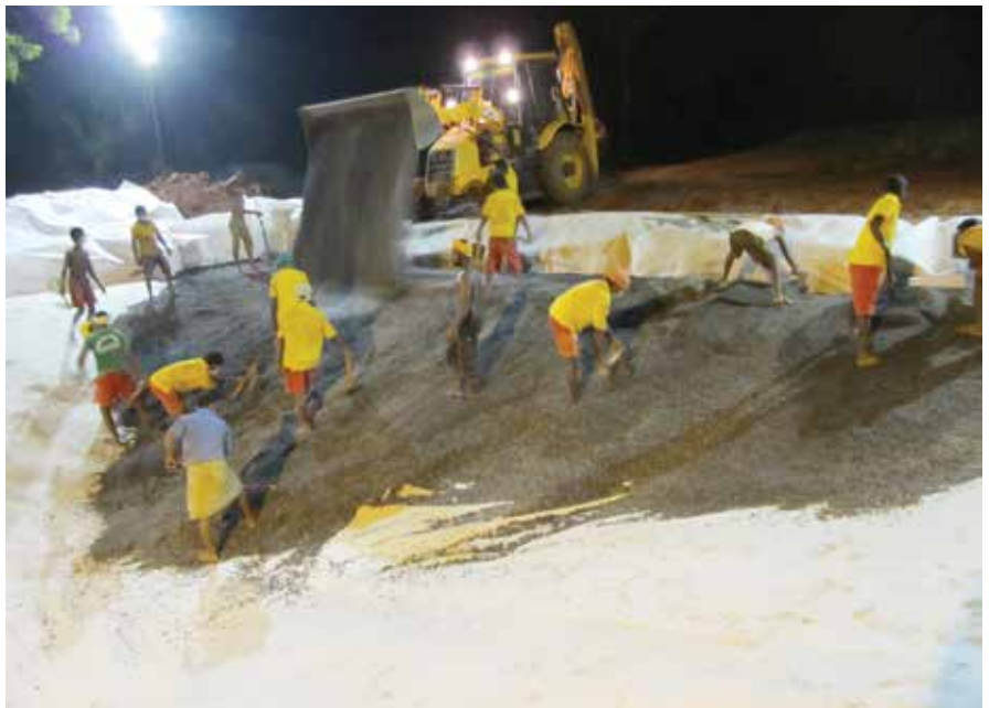
The sealed clay layer was covered with a protective layer of white geotextile, and then with a thick layer of granite chips.
