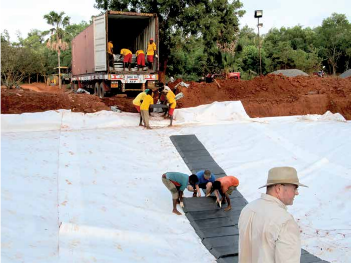
Laying compacted clay slabs on a geotextile under layer in one of the six mini test ponds at Matrimandir
